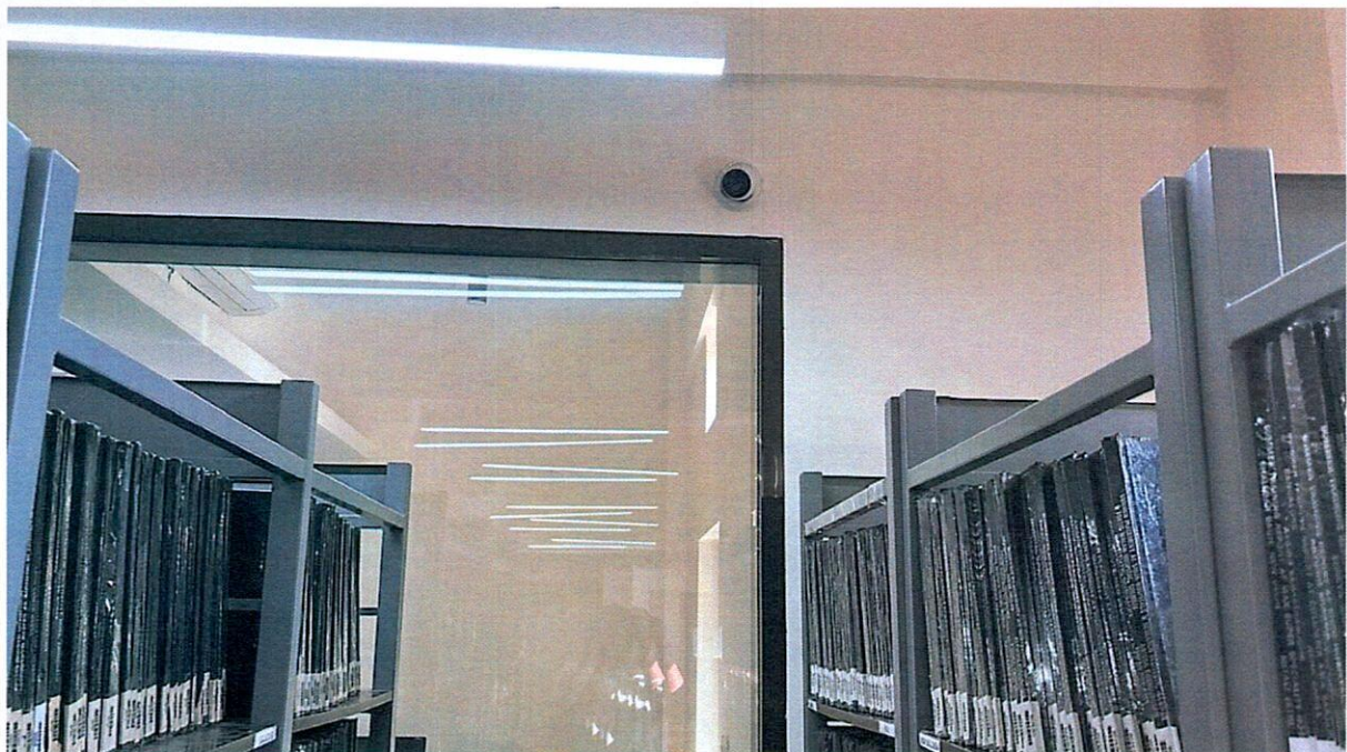
CCTV AT THE LIBRARY
