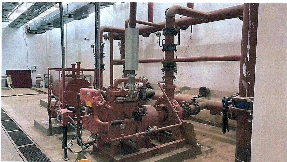
FIRE FIGHTING SYSTEM – WATER PUMP SETUP
