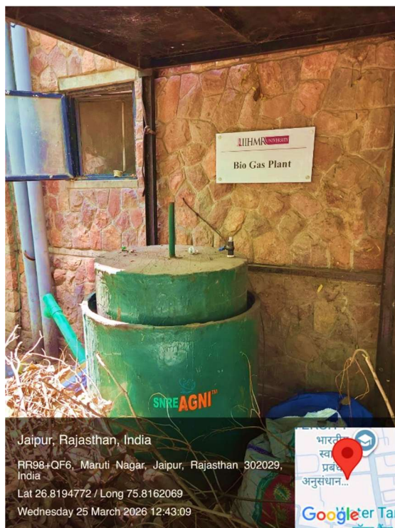
Biogas plant behind the Mess Area
